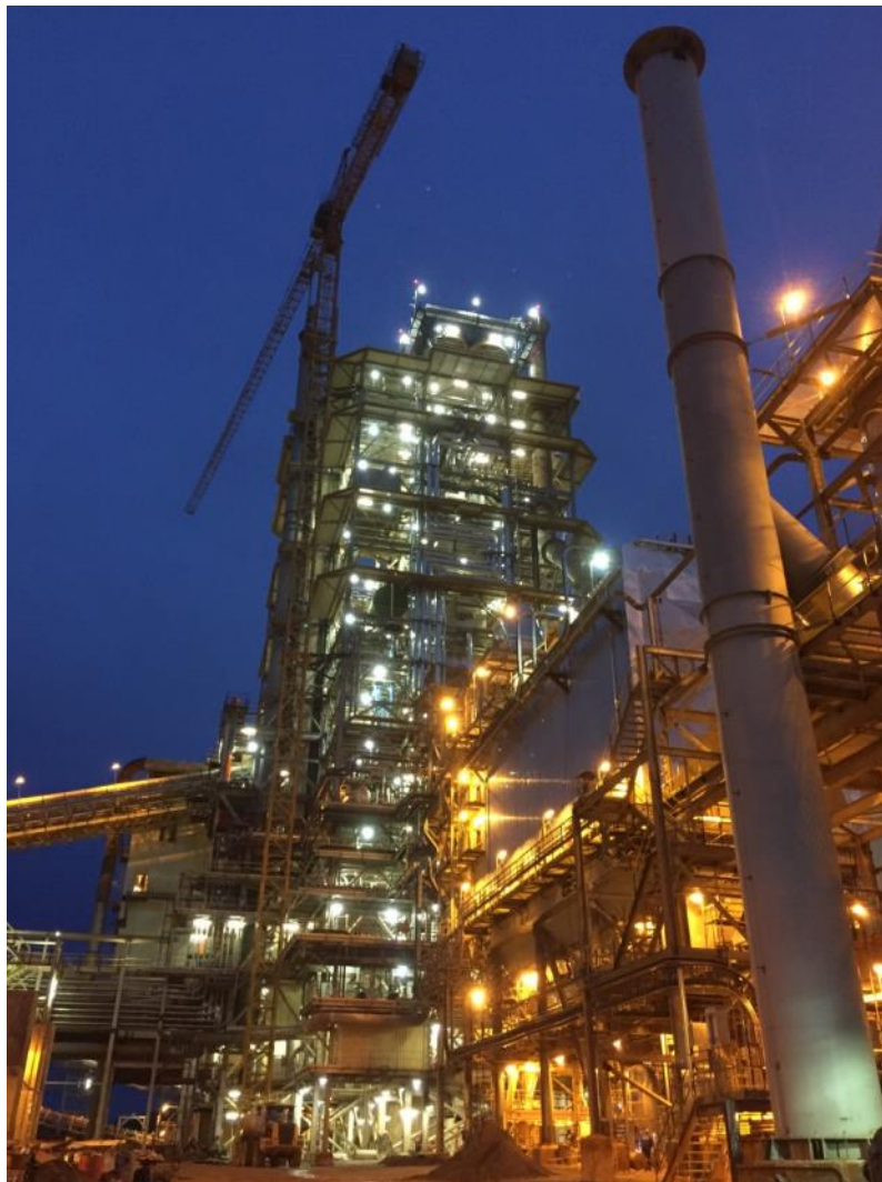
First Quantum's new ISASMELT™ plant at Kansanshi
