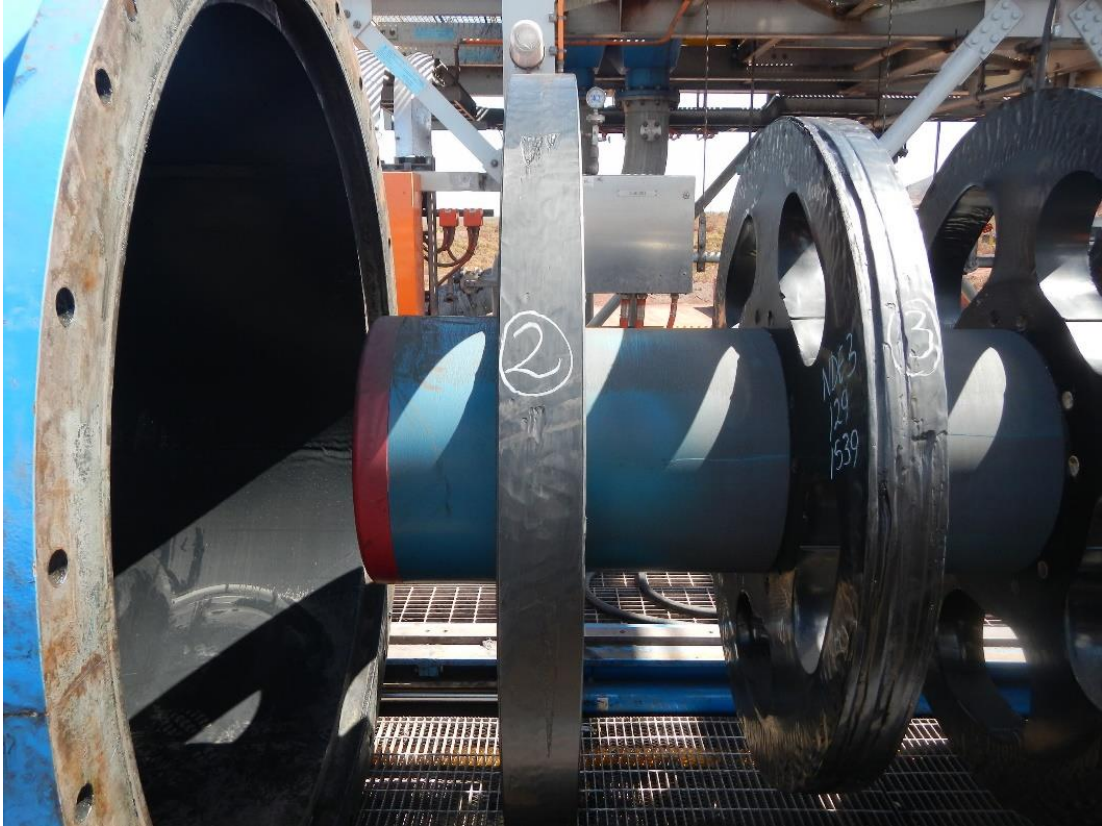
Figure 8: SDD installed at Zone of Compression
